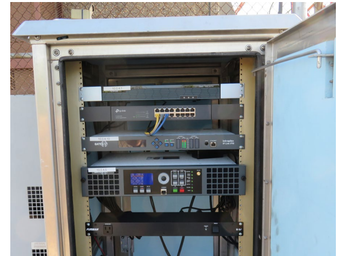
Rack from typical node
